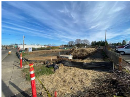
February 9, 2021: Hwy 213 at 211 is the future site of the Colima Apartments, a 36 unit complex.
