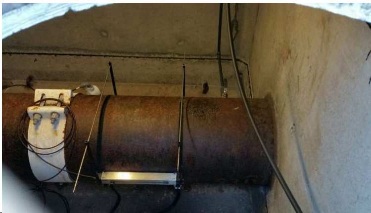
Figure 5 – New Ultrasonic Flow Meters at the Water Plant have allowed us to measure total water usage of the town to within approx. 5%. This will greatly assist water audit efforts and the ability to Master Plan the system beginning in 2019.
