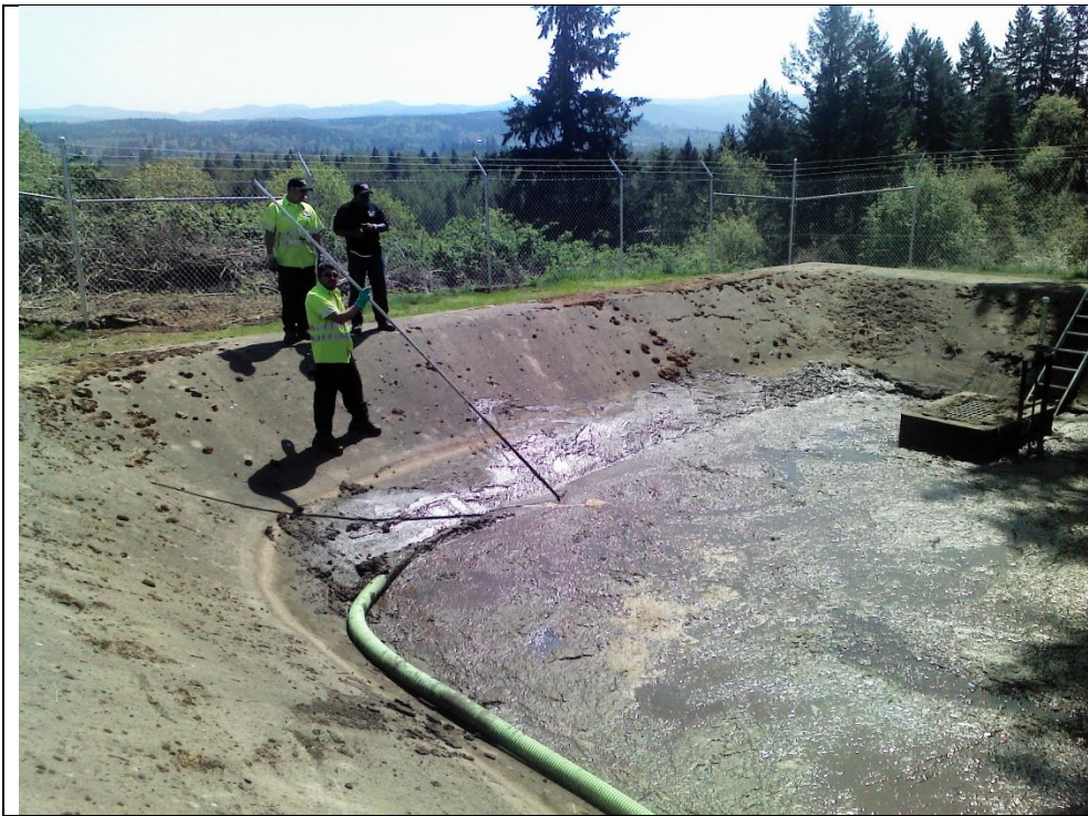
Figure 2 – Contractor River City Environmental begins the process of cleaning out the basin. Five trucks ran continuously carrying this “sludge” away. The sludge is made up of everything the Water Plant filters from our drinking water before sending it to town for our consumption.
