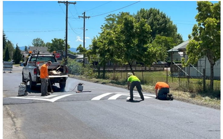
City Street Maintenance Crew puts the finishing touches on the West Lane paving project
