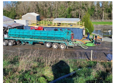
Biosolids Removal is now a continuous operation at Molalla's Wastewater Treatment Plant
