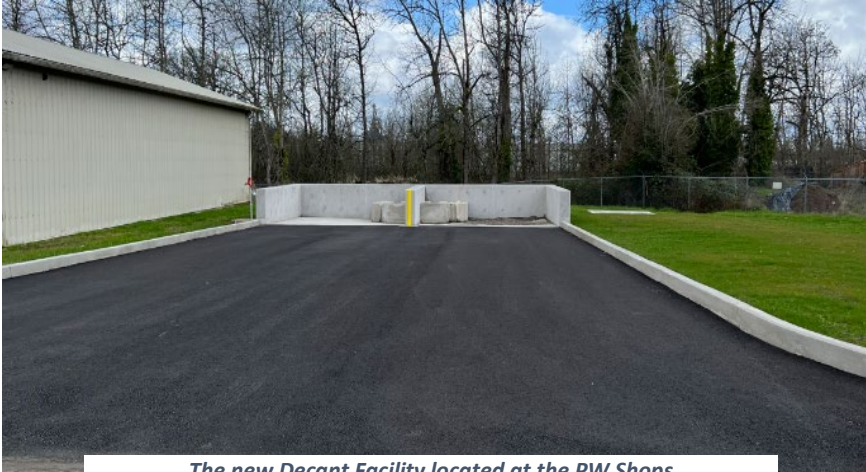
The new Decant Facility located at the PW Shops
