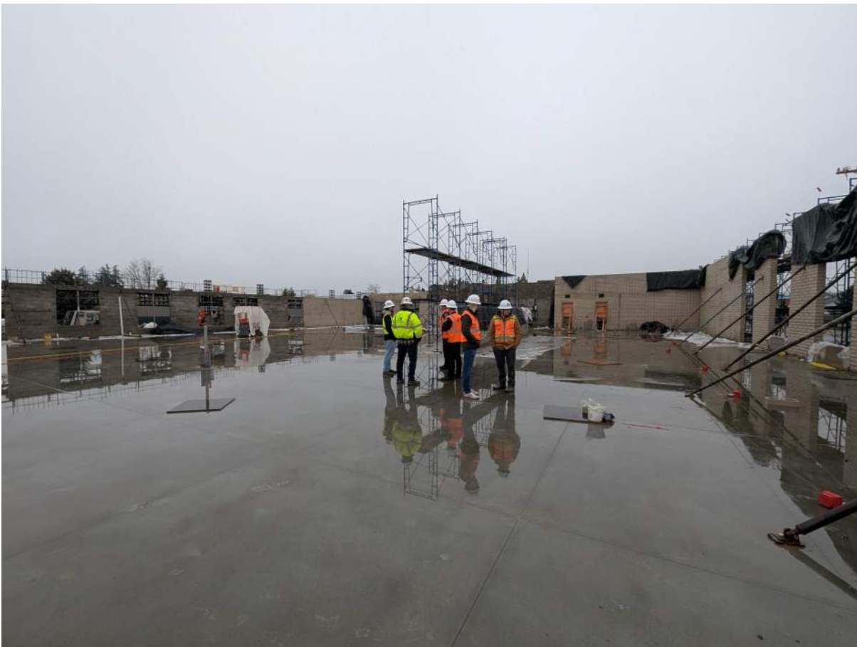
Figure 1- 12.12.2024- Team walk post OAC meeting- final interior slab and masonry wall progress
